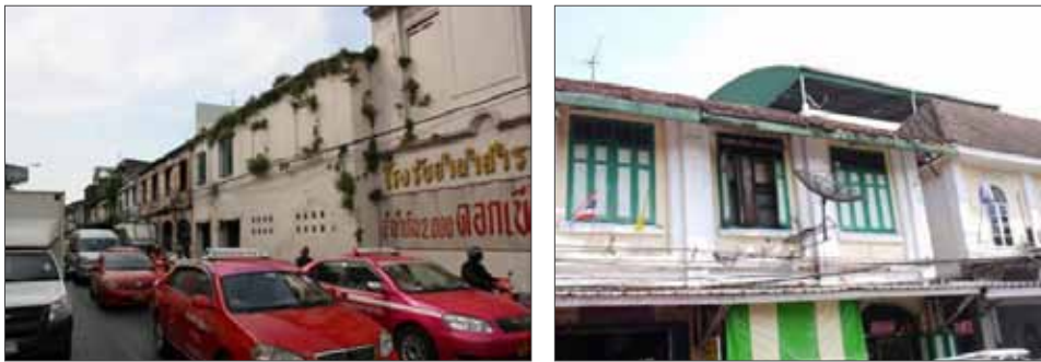
Figure 5. The heritage buildings with altered structure to fulfill the growing needs of its occupants in the Bangkok old town area. Photographs by the author.
