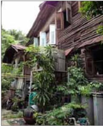
Figure 6. In this picture of a Crown Property Bureau structure, the building is in very poor condition due to lack of awareness and preservation by the tenant and the CPB. It represents a loss of an old memory and heritage. Photograph by the author.
